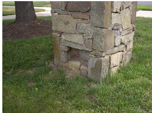
Damaged Stone Monument
