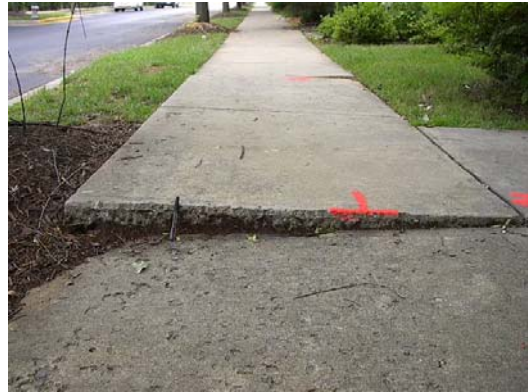
Concrete Tripping Hazard
